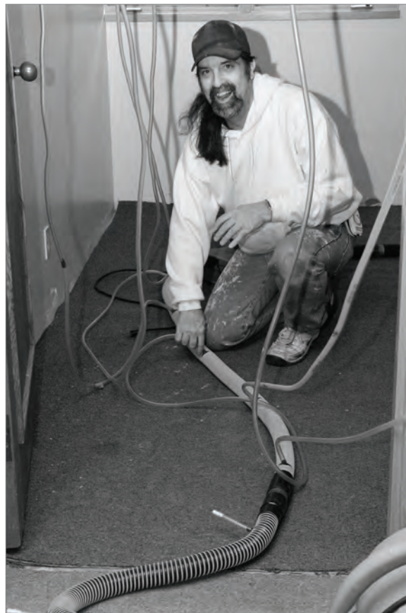
Disaster recovery crews from Kennedy Restoration injected air into wall and ceiling cavities to speed drying.
